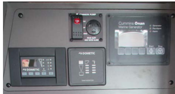
Water alarm; generator control panel; climate control panel; and waste/water tank level indicators
