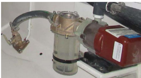
Air conditioning pump, strainer, and valve
