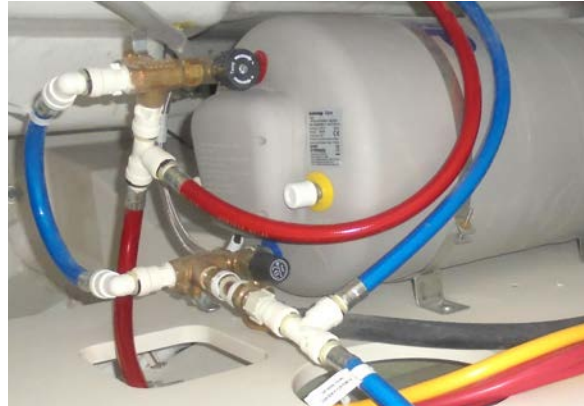
Water heater (typical)
