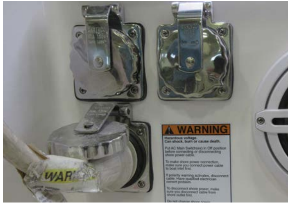
Shore power and cable TV inlets
