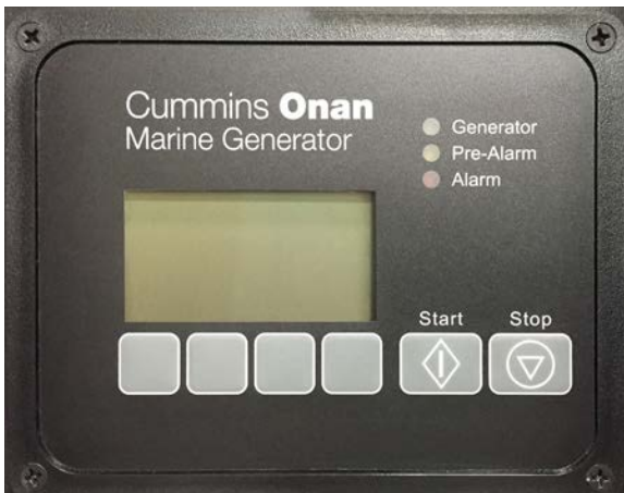
Remote generator control panel, in the head compartment electrical cabinet
