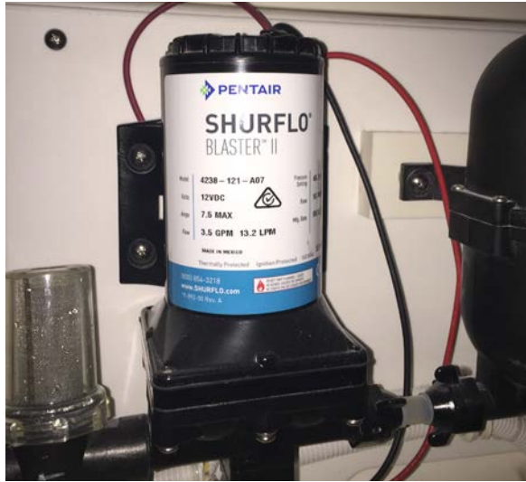
Raw water strainer (left) and pump (typical)
