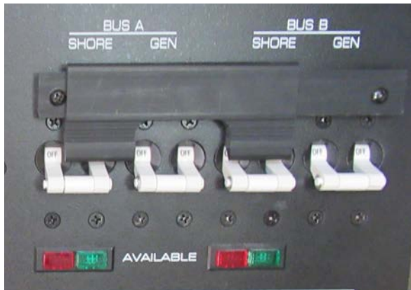
Shore power and generator indicator lights, on the AC distribution panel (typical)
