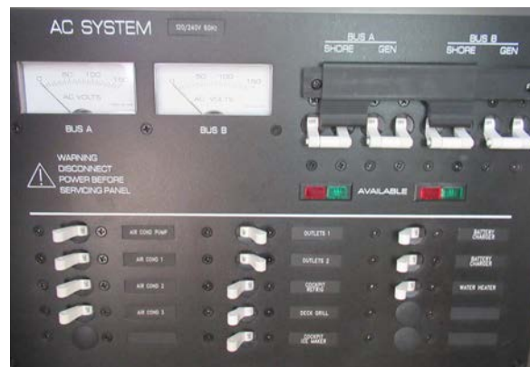
AC distribution panel
