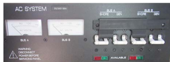
Shore power and generator select switches and polarity indicator lights
