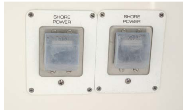
Main shorepower inlets in the port aft lounge seat base
