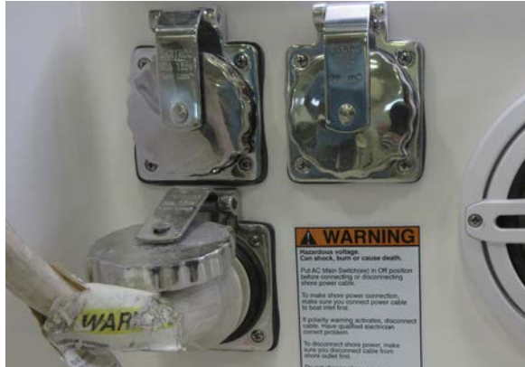
Shore power and cable TV inlets
