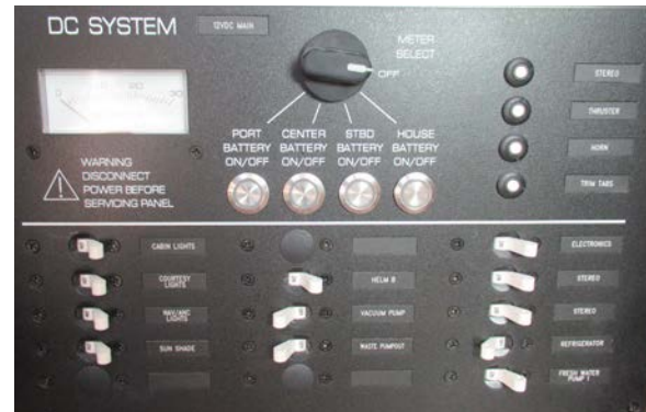
DC distribution panel
