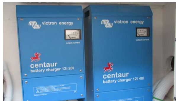
Battery chargers (typical)
